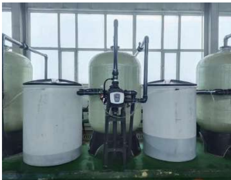
Water Softening Equipemnt for Car Washing
