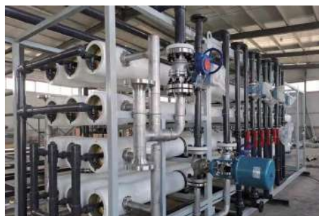
35 t/h Desalination Plant
