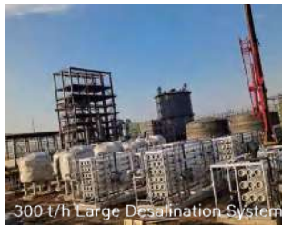
300 t/h Large Desalination System
