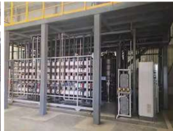
Auto Parts Plant Water Treatment Equipment
