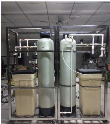
Water Softening Equipemnt for Car Washing
