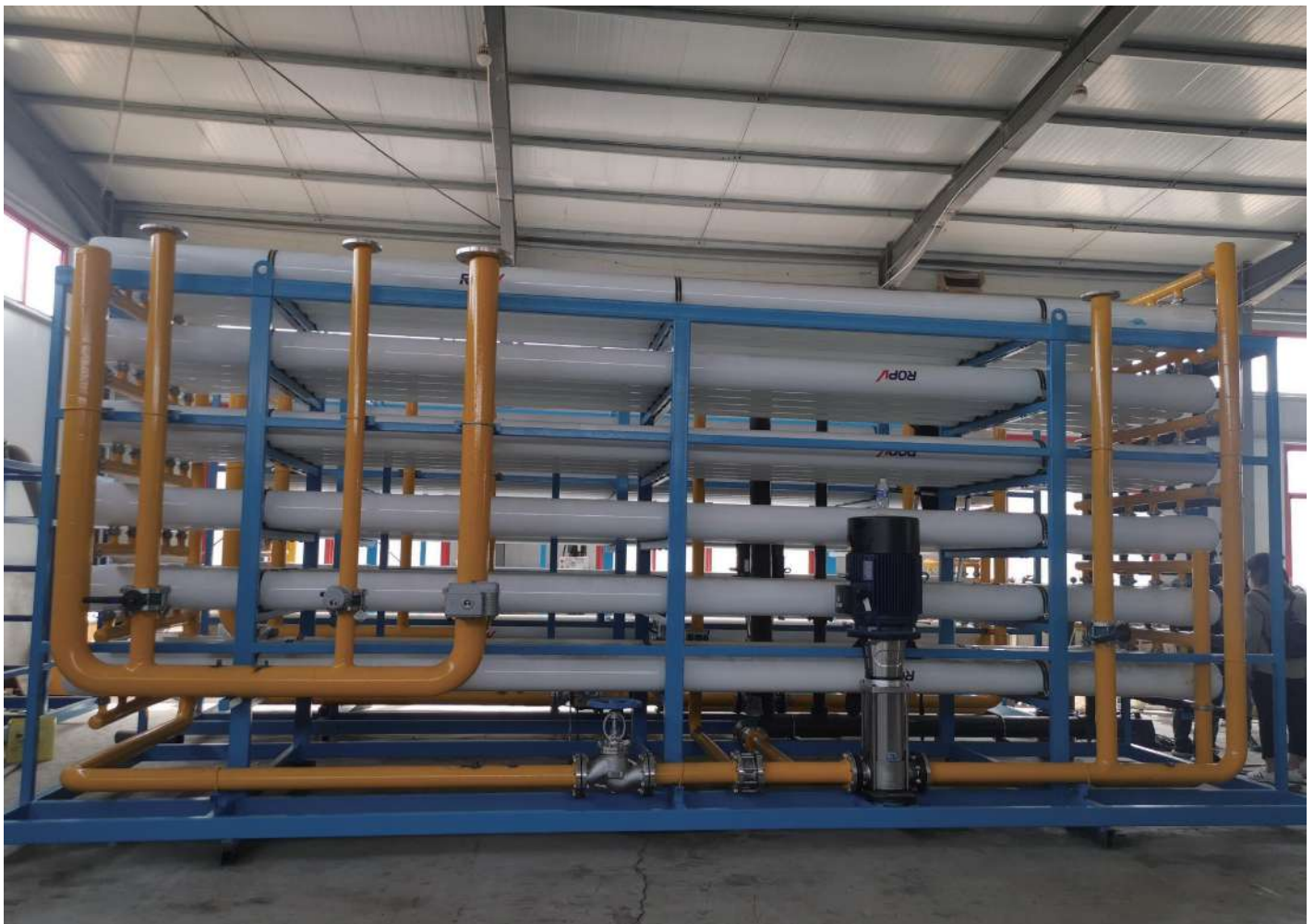
Mine Water Treatment Plant
