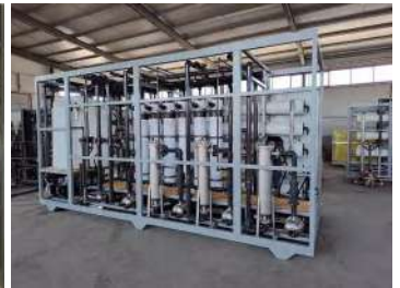
Ultrafiltration + Reverse Osmosis Equipment
