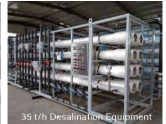
35 t/h Desalination Equipment
