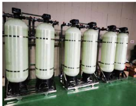
Water Softening Equipemnt for Car Washing
