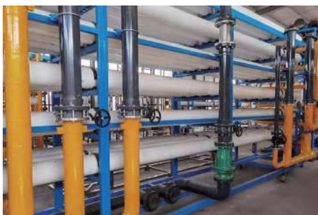
140 t/h Reverse Osmosis Equipment
